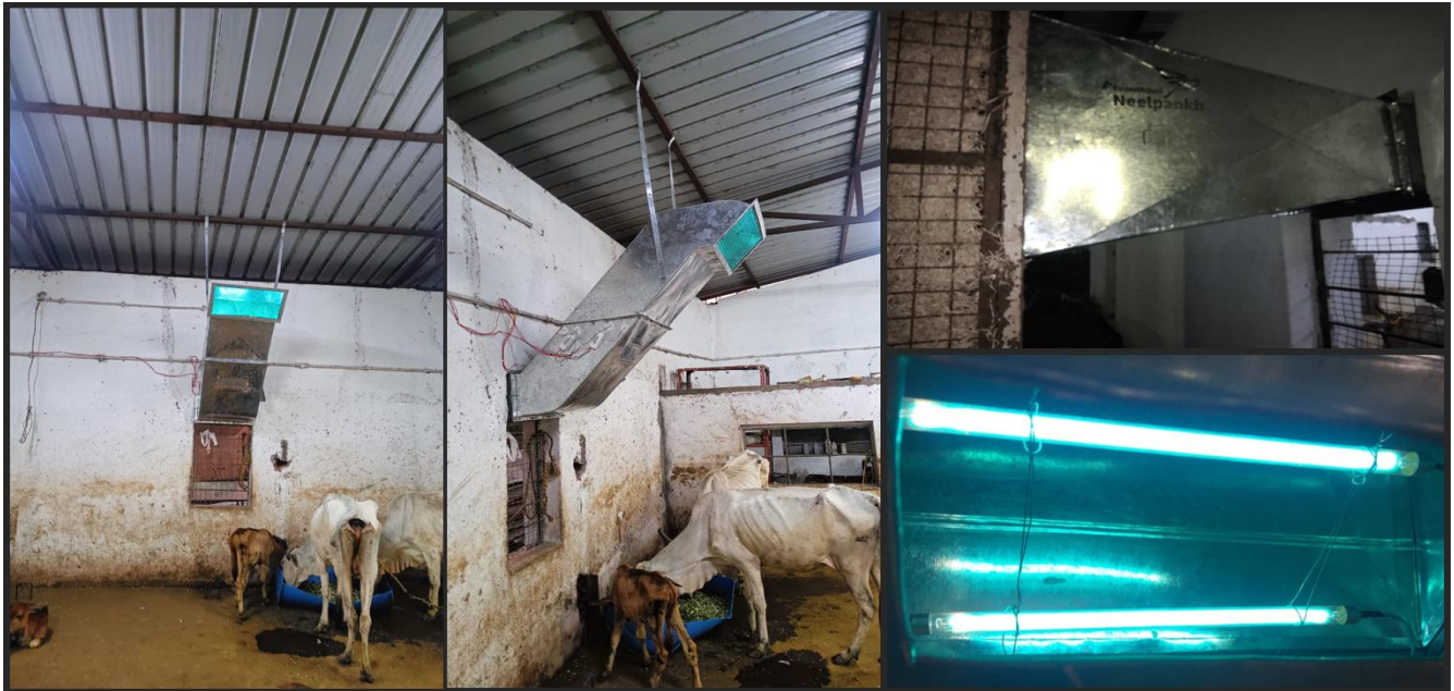
Fig. 4 Ducting setup in the cattle shed with UV light.
