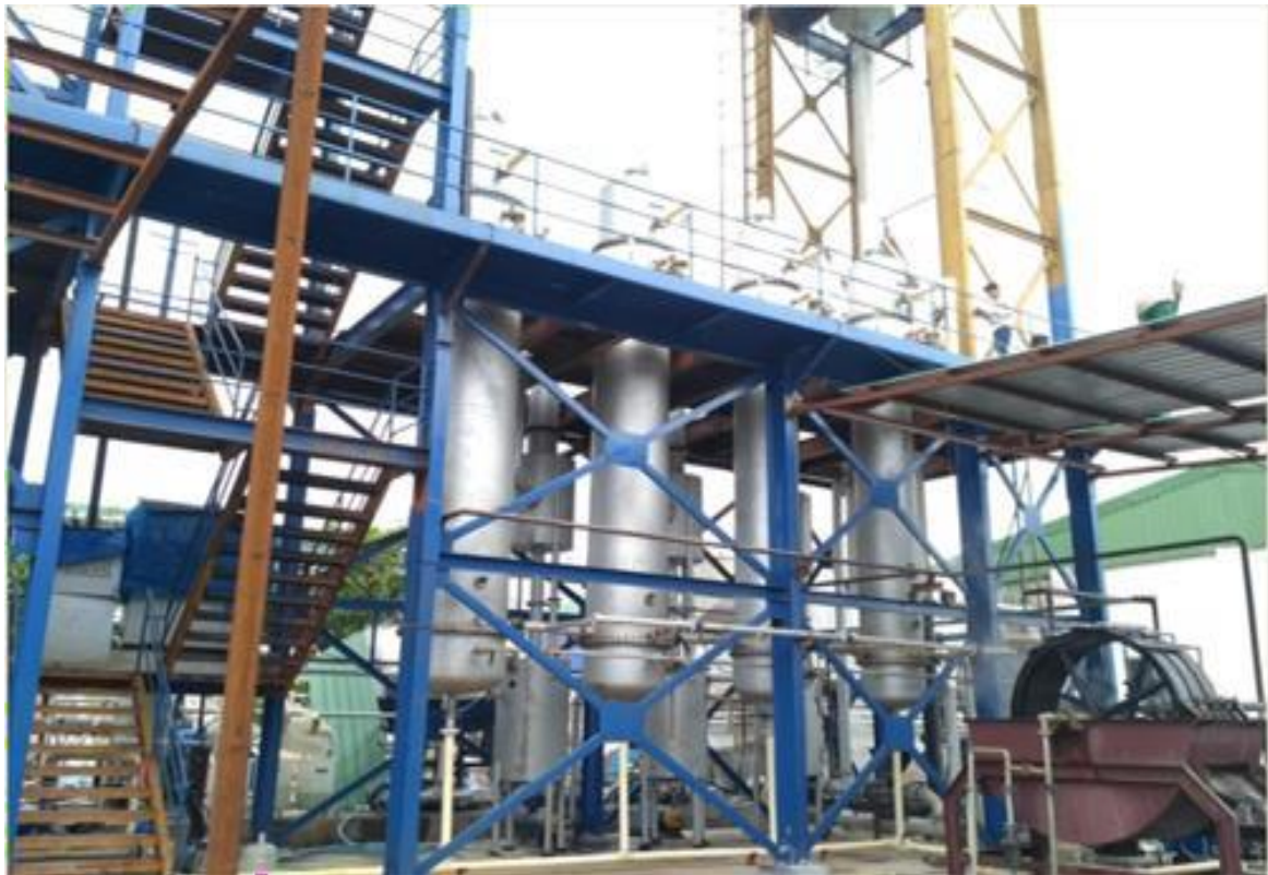
Fig 7: Effluent Uniformly passing through Evaporator
