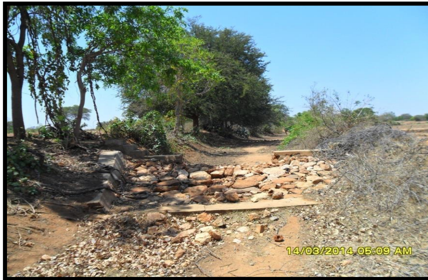
Picture – 2: Check dam in the Area (damaged)
